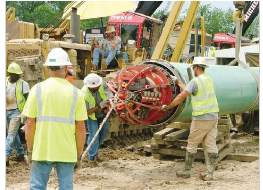
Workers use specialized equipment to make certain sections of the pipe are aligned. DAVID AMEY/Circleville Herald
